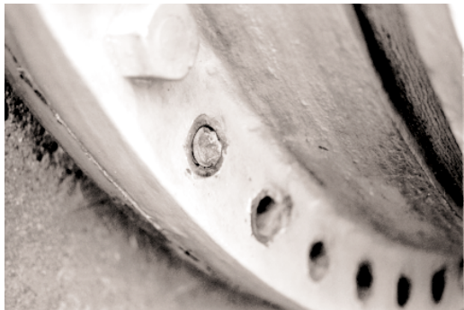
Figure 9. Dezincification of Brass Containing a High Zinc Content (Reference 12)
